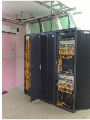
Fig. 11 The CO room showing the OLTs rack and the ODF
