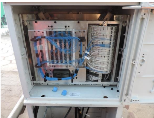
Fig. 13 Level-1 splitter inside the FDT
