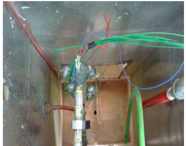
Plate (2.b): Top view of the water heating and circulation tank
