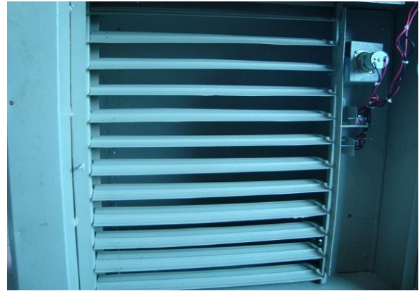
Fig 13: Louver of Fan and Filter Unit
