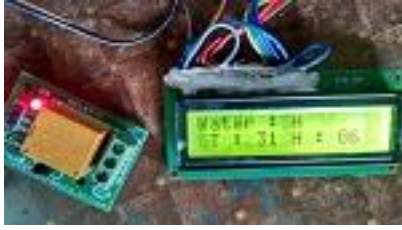
Fig 11. Displaying the water and humidity levels
