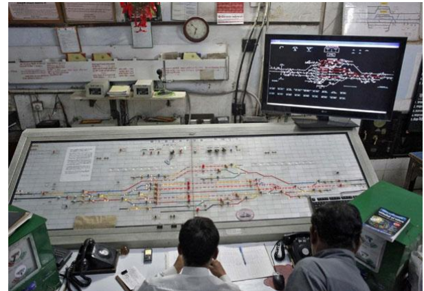
Fig 1: Route Relay Interlocking System (Source: How does the Inside of Control Room of Indian Railways Look Like.)
