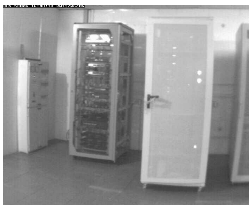
Fig 6: Faulty image indicating the smoke intrusion
