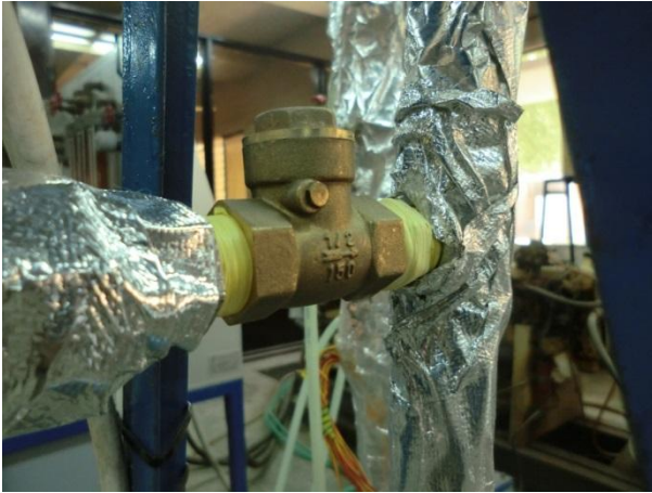
Plate (2): Check valve connected directly before the pipes bridge.
